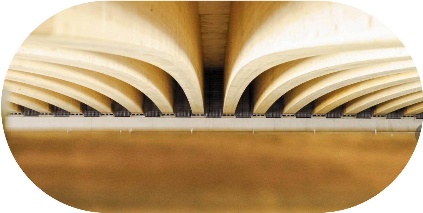
Bouygues Construction, via its subsidiary VSL International, was involved in the construction of the world's first-ever prestressed timber bridge in Switzerland
