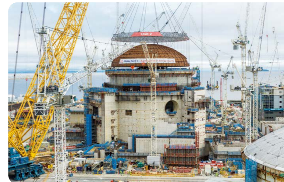
UNITED KINGDOM – Hinkley Point C EPR power plant, built by the BYLOR Joint-Venture (Bouygues Travaux Publics, Laing O'Rourke). Once in operation, the Hinkley Point C EPR will help to avoid emissions of around 9 MT of CO 2 per year, namely twice the annual emissions of Bouygues Construction.
