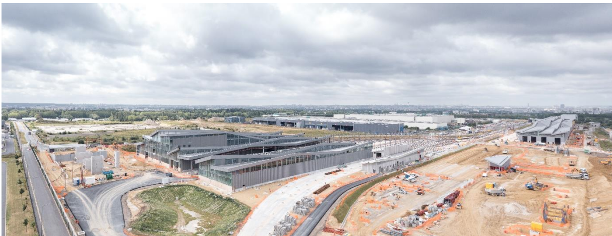
The future operations centre for metro lines 16 and 17 of the Grand Paris Express ©Nicolas Grosmond
