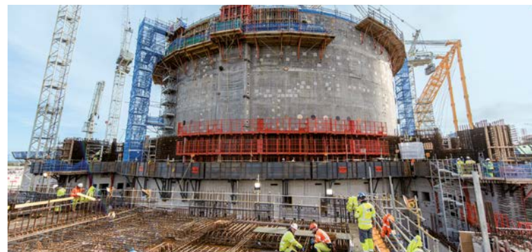
UNITED KINGDOM – Bouygues Travaux Publics, as part of the Bylor consortium, is building the structural elements of the two EPR reactors for the future Hinkley Point nuclear power plant.
