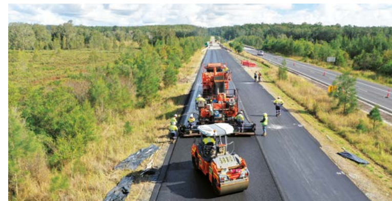
AUSTRALIA – A Colas Australia team lays SMA10-graded asphalt on a road near Clybucca, New South Wales.
