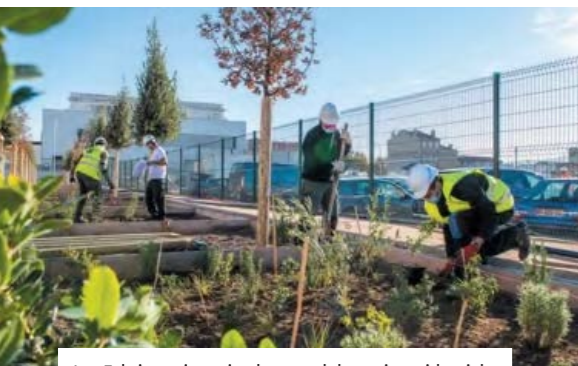
Les Fabriques is a mixed-use and dynamic residential neighbourhood built on a former brownfield site in Marseille. To encourage the growth of vegetation, 85 species of local tree and shrub were planted there.
