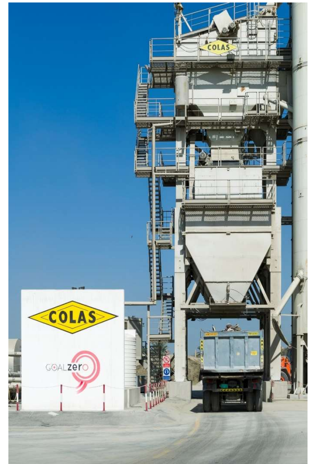
Asphalt plant - Dubai
