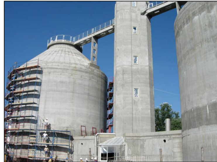
ALTERRA water treatment plant, Hungary
