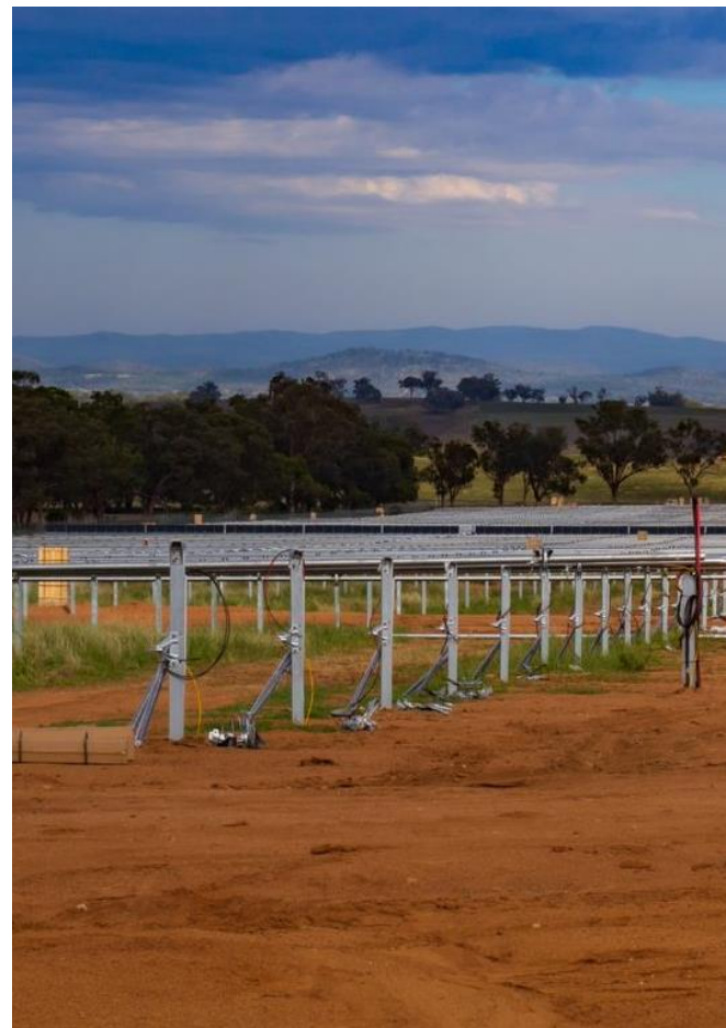
Bouygues Energies & Services – Suntop solar farm – Australia
