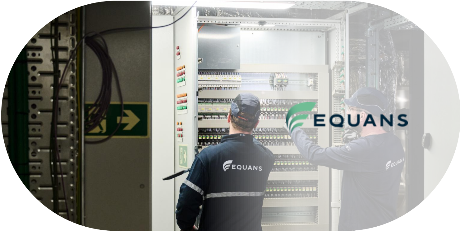
Energy efficiency and smart buildings at Namur regional hospital (Belgium) by Equans
