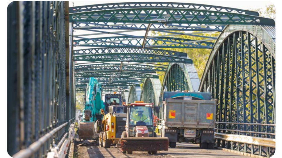
AUSTRALIA - Colas Australia rehabilitated the Burnett river bridge in the city of Bundaberg, Queensland. The work was planned meticulously and carried out day and night, with scheduled closures and enhanced safety measures, to restore the 120-year-old structure to its full function.
