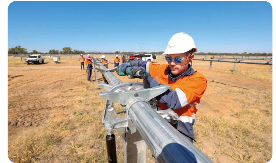
AUSTRALIA - In Culcairn, Australia, Bouygues Construction Australia and Equans Solar & Storage are building the largest solar farm ever built by the Group. This large-scale project, carried out as part of a joint venture on behalf of Neoen, will eventually be used to power 155,000 homes.
