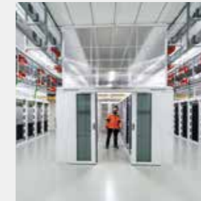
The CERN data centre in Switzerland, built by Equans
