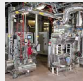
Environmentally friendly cooling system and a high-temperature heat pump at the Ennstal dairy farm in Austria, installed by Equans
