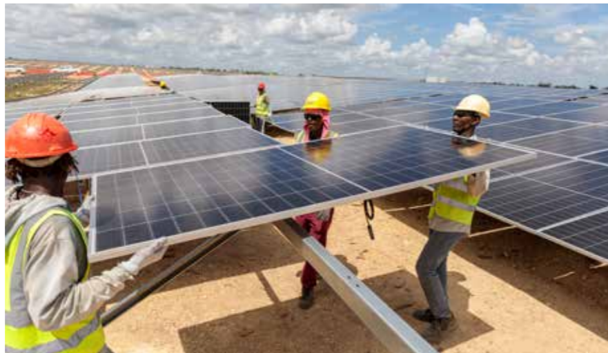
DOMINICAN REPUBLIC - Equans Solar & Storage is building several solar farms in the Caribbean nation.
