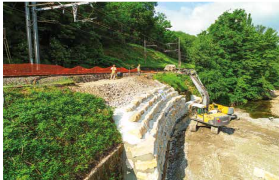
FRANCE - Hydraulic and environmental engineering: gently sloping riverbank upstream, floodplain and natural spaces to avoid disrupting beaver populations downstream, and confluence with the Couzon river to expand the Gier's meander belt.
