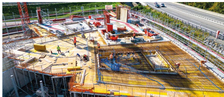
SWITZERLAND - At 131 Stauffacherstrasse in Berne, Losinger Marazzi (Bouygues Construction) is responsible for the development and construction of a hybrid timber-frame services building.
