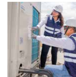
An Equans data centre in Peru
