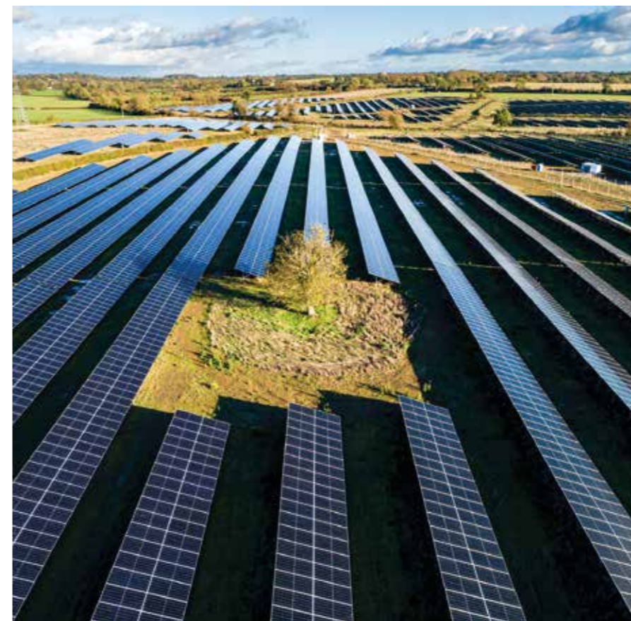
UNITED KINGDOM – The Fox Covert solar farm in Buckinghamshire will produce enough power to provide 7,500 households with electricity, helping to avoid 4,942 tonnes of CO 2 equivalent every year.
