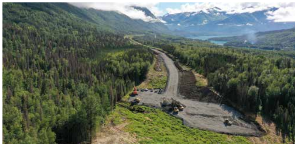
UNITED STATES – On the Kenai peninsula, in southern Alaska, Colas won a major contract to upgrade the Sterling Highway (resurfacing, creation of overtaking lanes and wildlife crossings, as well as a 15-km extension of the route).
