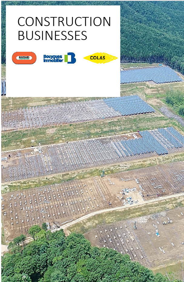
13.7 MW solar farm in Noheji, Japan
