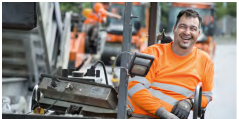
📷 Mohamed Boudemdani from Colas Nord-Picardie working on the A22 motorway in northern France.
