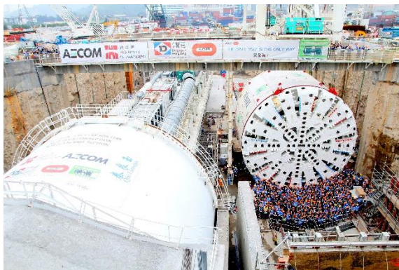
World's largest tunnelling machine, Tuen Mun – Chek Lap Kok tunnel worksite, Hong Kong
